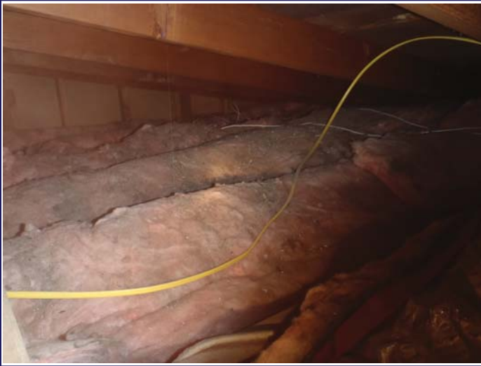
Loose electrical wiring in the attic area
