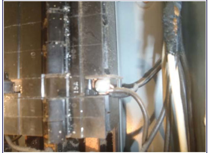
Double tapped 15 amp single pole circuit breaker in the sub panel
