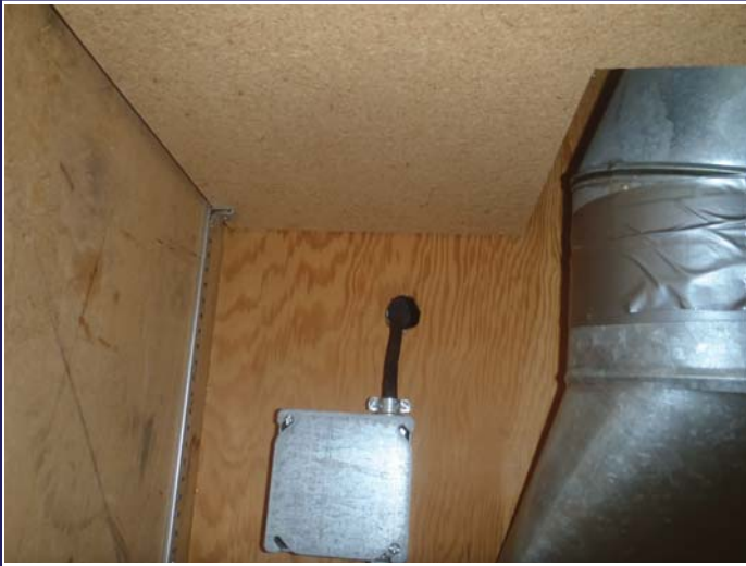
Unprotected electrical wiring in the kitchen cabinet above the stove
