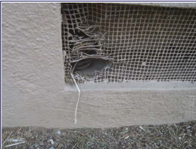
Broken foundation vent around the rear of the house
