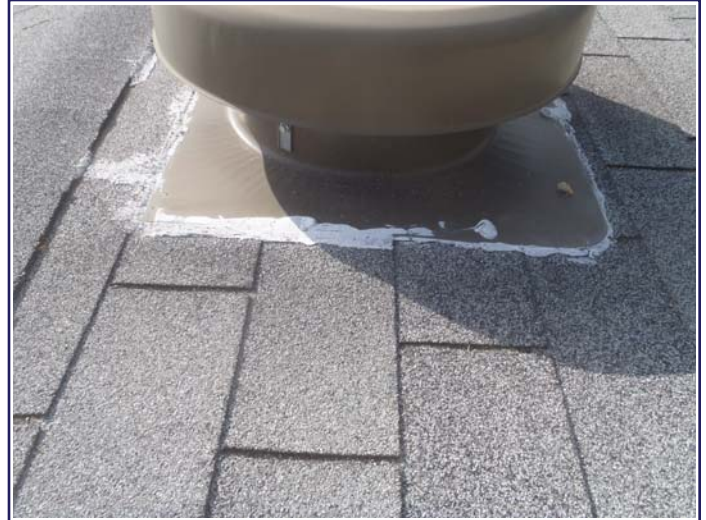
Attic fan/flashing above the rear of the house is not properly installed
