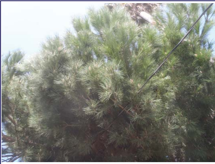
Main electrical cables in contact with tree branches
