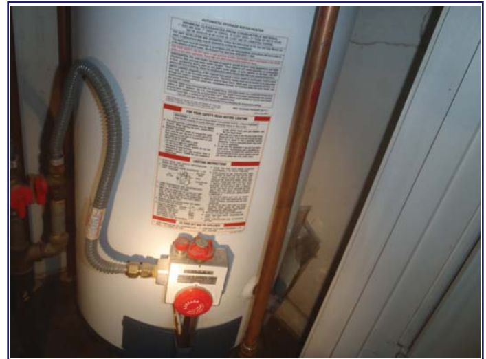
Water heater tank is not properly seismically strapped
