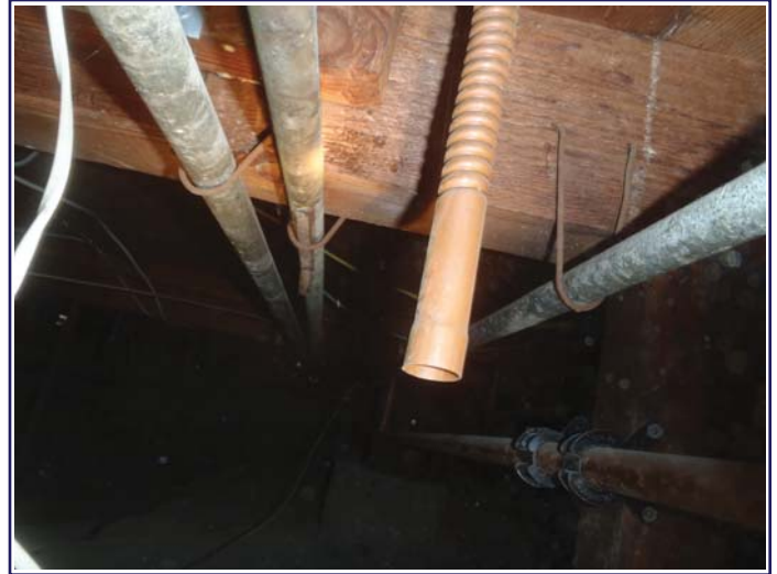
Discharge pipe for the water heater's TPR valve terminates in the sub area
