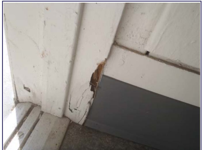
Damage to the bottom portion of the garage side door jamb/trim
